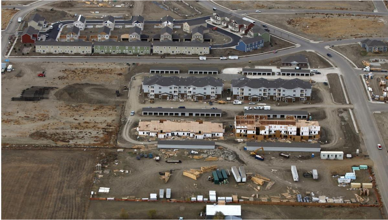
Figure 18. New residences being constructed in Williston, 2012. From The Atlantic , photo credit: Jim Urquhart, Reuters.
